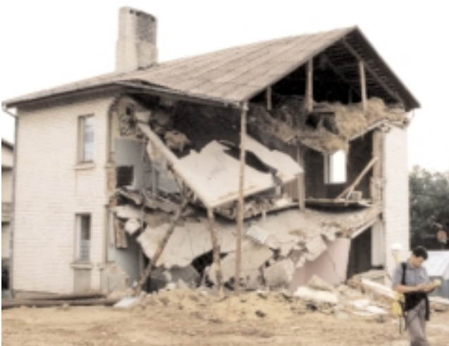
House damaged by sudden collapse of karstic cavity, Pasvalys.
