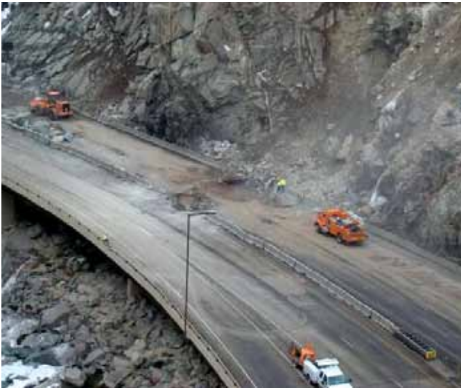
Aerial view of Glenwood Canyon, Colorado, rockslide onto Interstate 70, March 2010. Photo by CDOT, used with permission from the USGS.
