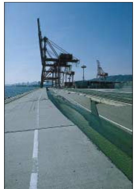
Figure 10. Damage to Maya Wharf caused by liquefaction-induced lateral spreading. The quay wall moved outward, causing formation of a graben. The seaward rail for gantry cranes is located on the quay wall, and the landward rail is located on a pile-supported wall behind a graben.
