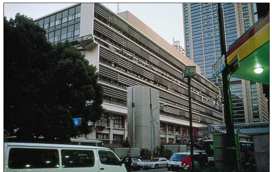
Figure 8. Collapsed sixth story in eight-story Kobe City Hall Annex, a reinforced-concrete building built in the 1960s. Behind it is the 16-story New City Hall, a 1980s steel-frame building that was not damaged and remained functional after the earthquake. (Photograph by Christopher Rojahn, Applied Technology Council.)
