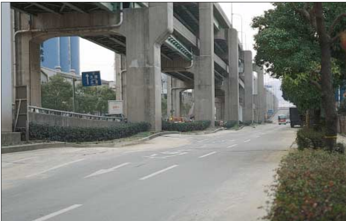
Figure 5. Differential ground settlement in artificial fill beneath the Harbor Expressway near Rokko Island. Postliquefaction consolidation caused ground to settle between bridge columns. Columns extend through liquefied zone. (Photograph by Carol S. Prentice, U.S. Geological Survey.)
