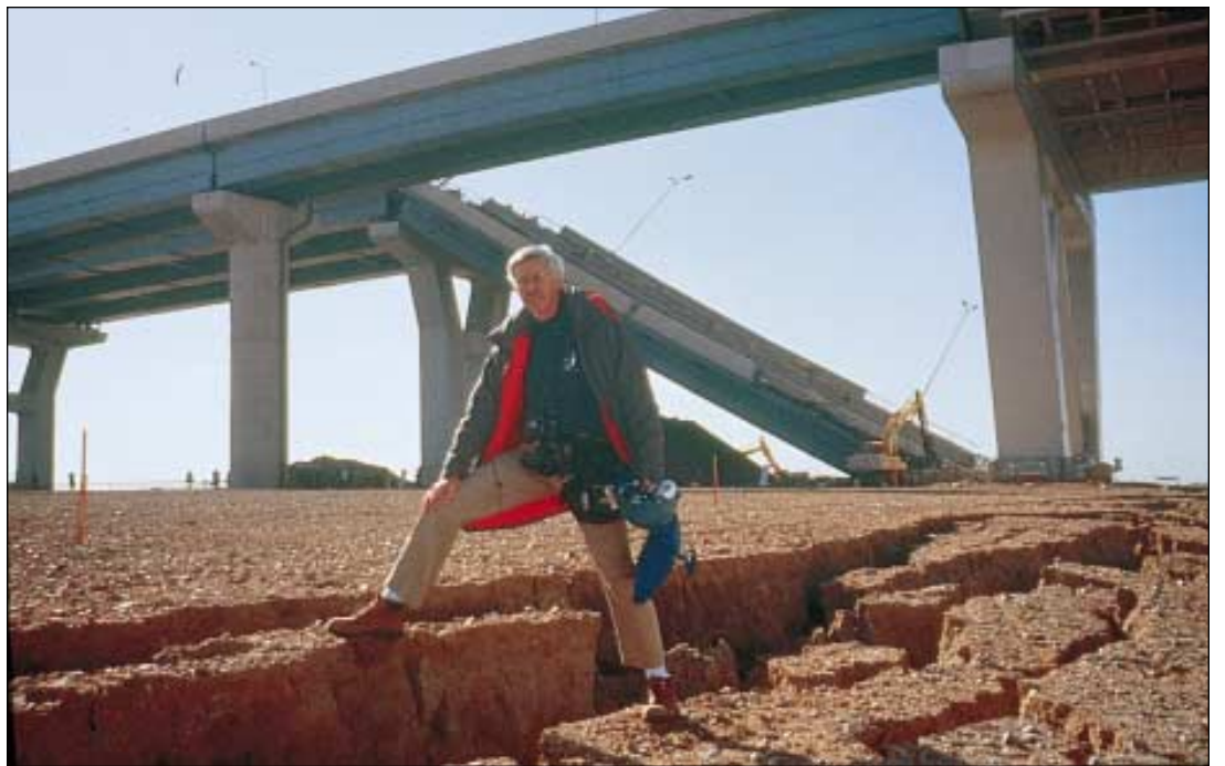
Figure 9. Nishinomiya Harbor Bridge where an approach span collapsed. Thomas D. O'Rourke of Cornell University stands astride ground crack caused by liquefaction-induced lateral spreading in bridge foundation.
