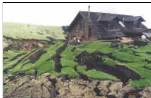
Figure 12. Reactivated earthflow near town of Aromas (see Fig. 2 for location), that cut natural gas service to 60,000 Santa Cruz County residents on April 23, 1998. Photo by W. R. Cotton.
