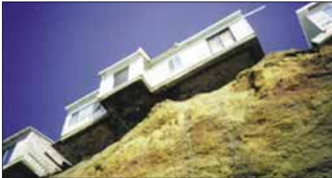
Figure 10. Doomed houses on Esplanade Drive, Pacifica, perched on retreating sea cliff, from beach below. Photo taken April 1, 1998, by K. R. Lajoie.
