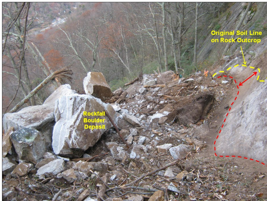
Figure 3-13. Displacement along the scarp of the debris slide developed here along the contact between bedrock and pre-existing rocky colluvium overlain by boulders from the November 14, 2012 rockfall event. The displacement is shown by the distance between the yellow and red dashed lines. 2012/11/19 NCGS photo.
