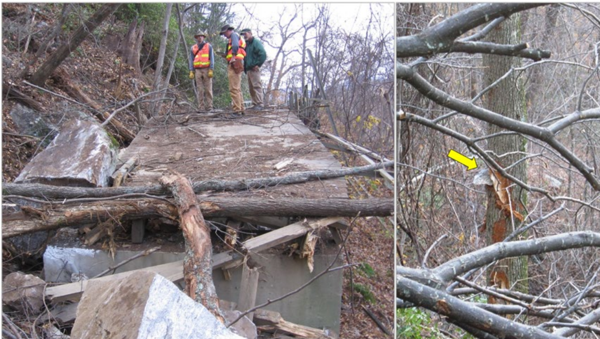
Figure 3-16. Left. Severe damage to the footbridge on Hickory Nut Falls trail caused by rockfall and trees downed by the rockfall. 2012/11/19 NCGS photo. Right. Arrow points to a rock projectile from the November 14, 2012 rockfall imbedded into a tree below the Hickory Nut Falls trail. The rock fragment is about 2.5-3.0 m above the base of the tree. 2012/11/19 NCGS photo.
